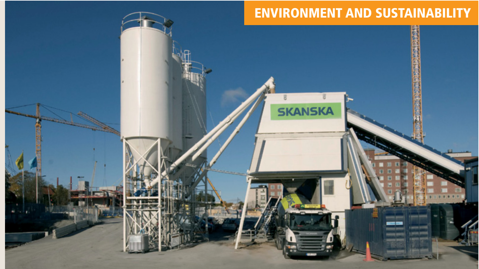
The concrete plant established on the construction site provides the project with concrete and reduces the number of trips by a total of 20,000.
