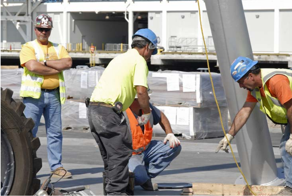
Project Superintendent, Mike Maione (left), supervises installation of the final shade structure support. Photograph by Julienne Schaer
