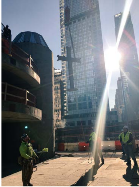
Photo 3 Caption: The temporary cross that was placed on top of St. Nicholas Greek Orthodox Church and National Shrine at the topping out ceremony on November 28, 2016.
